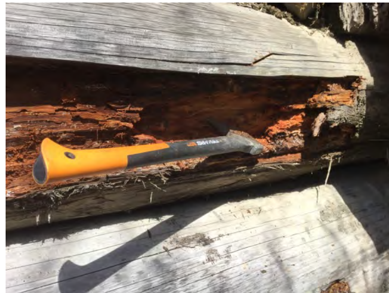
Log ballast wall rotten but still functional
