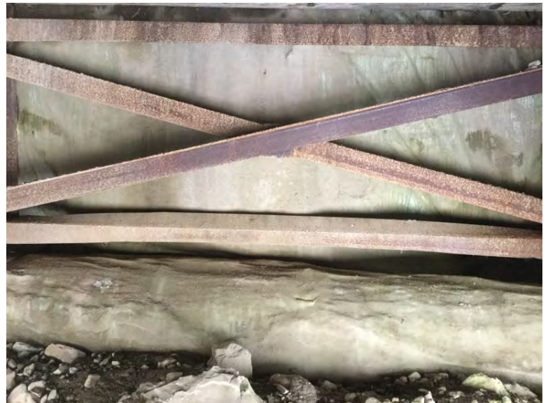
Bottom chord at left bank bent
